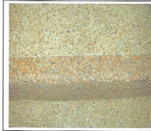
Mortar Paste system used to improve the steps and risers at this hotel with two colors for safety.
